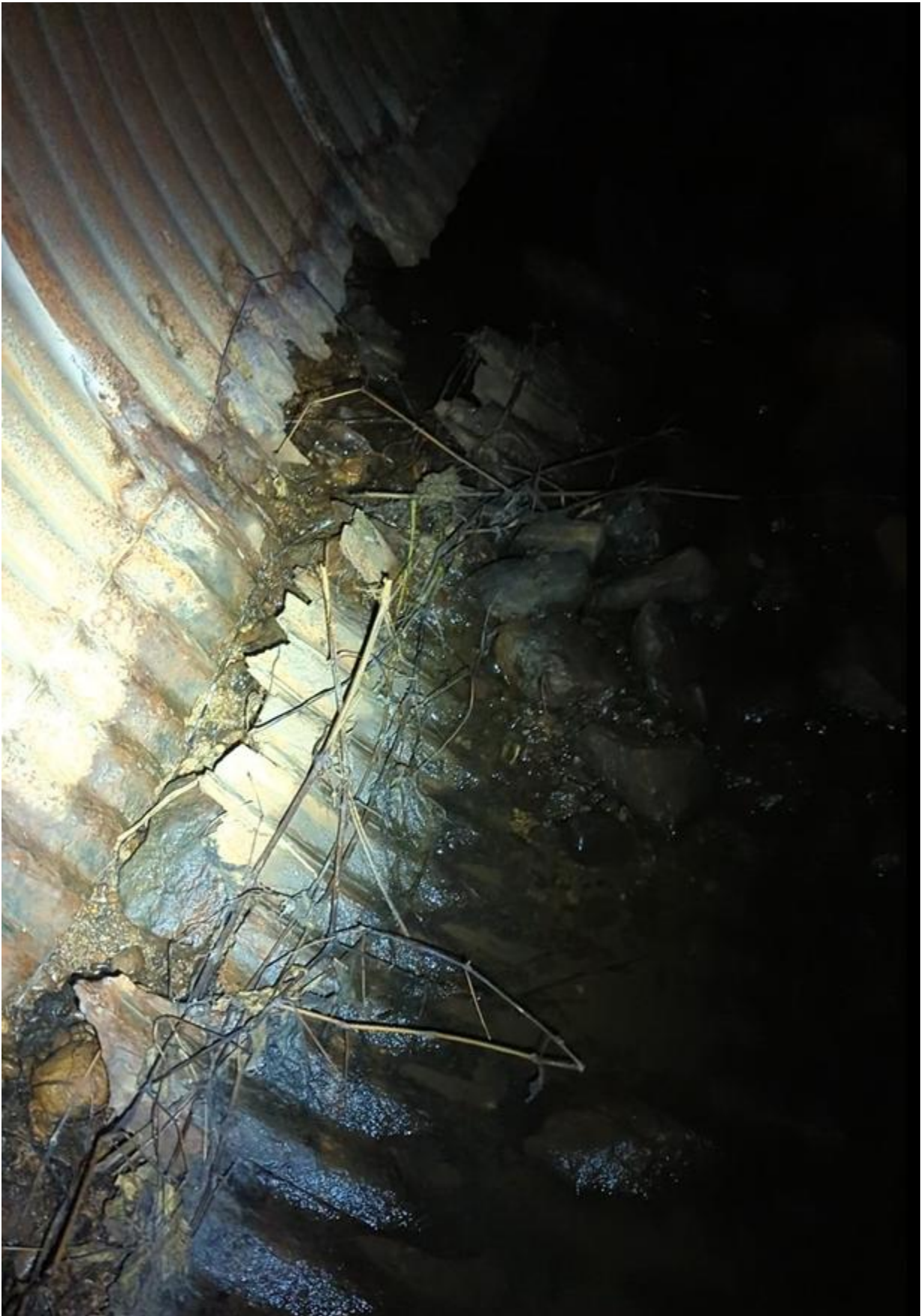
Eroded pipe bed
